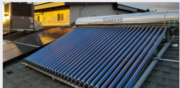
Solar Water Heating
